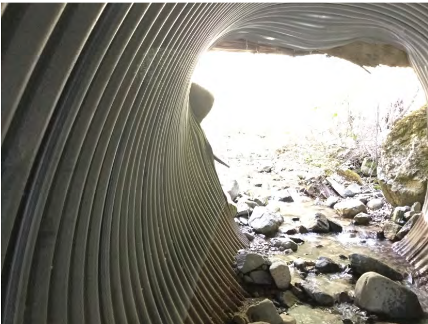
Sidewall damage at inlet
