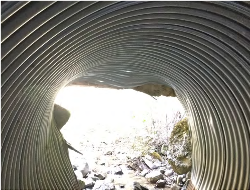
Damage to roof at inlet
