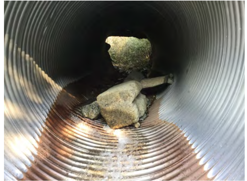
Material being washed into the culvert
