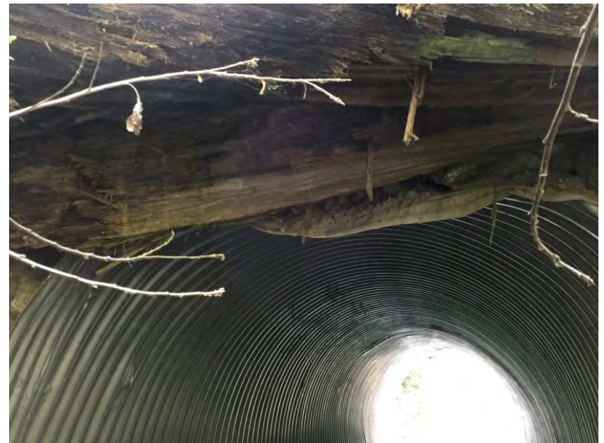
Damage to inlet from failing log fender
